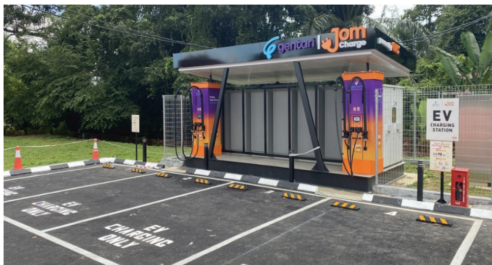
Gambar 3: Stesen EVCS Modular Mudah Alih dengan Sistem Simpanan Kuasa Bateri di Hentian Sebelah Behrang (Arah Utara), Lebuhraya Utara Selatan Image 3: A Portable Modular EVCS, with Battery Power Storage System at the Behrang Lay-by (North Bound), North-South Expressway
